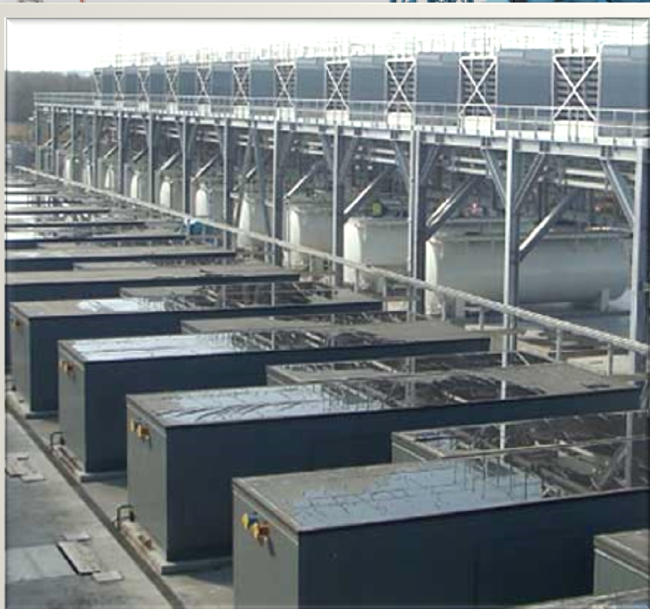
The equipment yard at the Google data center in Belgium features no chillers. (Photo from Google) b.
